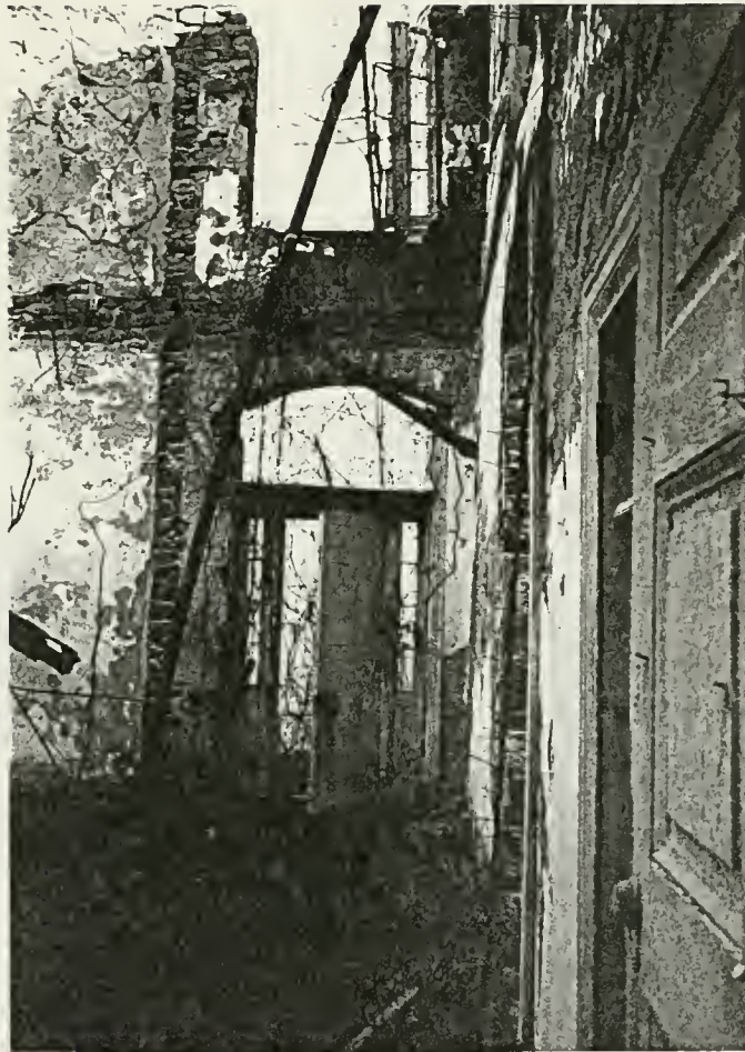
Figure 23: Second story plumbing for bathroom above central hall, leaning towards interior wall
